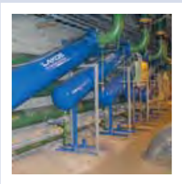
River Water Intake Central TN
